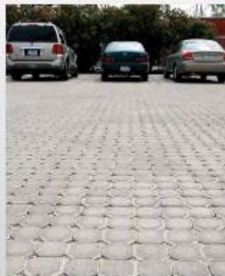
Rainfall soaks through permeable pavement and into the ground below in this parking area in west Des Moines, Iowa.
